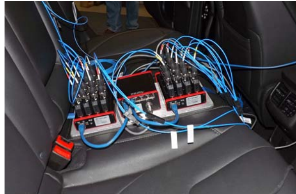
A 32-channel Titan DAQ system for standard seat and instrument panel NVH data collection
